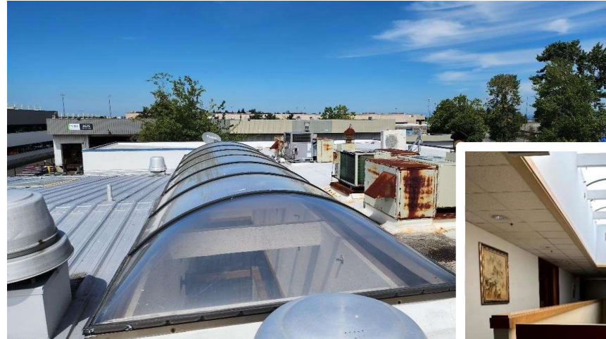
Aging Skylights Leak Water and Heat
