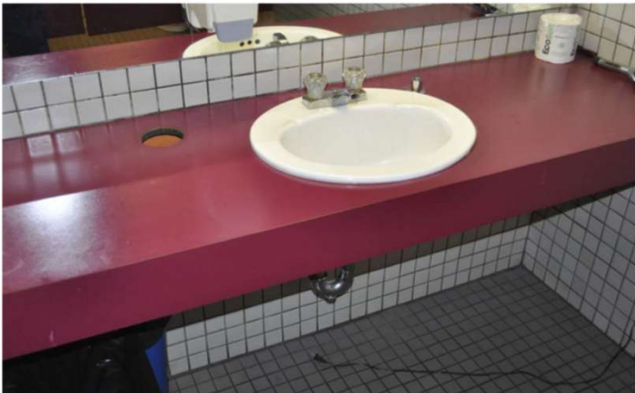
Restroom Fixtures and Surfaces Unhygienic Water Wasting Fixtures
