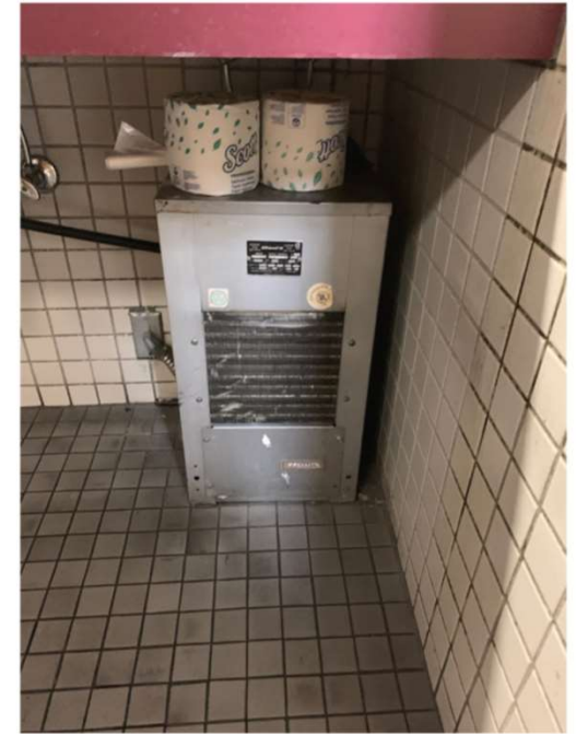
Inefficient or Broken Water Heaters
