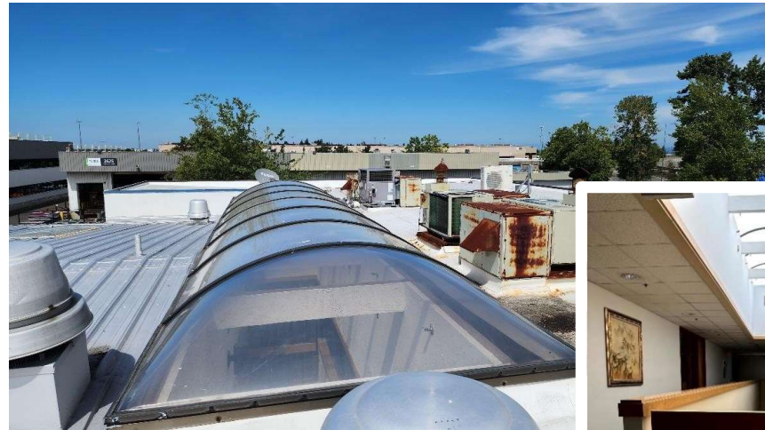
Aging Skylights Leak Water and Heat
